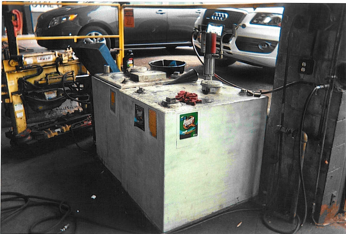
PHOTOGRAPH 2 – View of the two above ground storage tanks for new and used motor oil located in Bay 4. There is no drive in access to Bay 4. Equipment for tire mounting and balancing and a brake lathe are also in the Bay.
