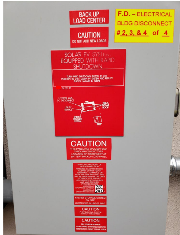
2 ND PANEL – EXTERIOR PLACARD OPTION 2: Combined Exterior Placards on a Panel/Enclosure
