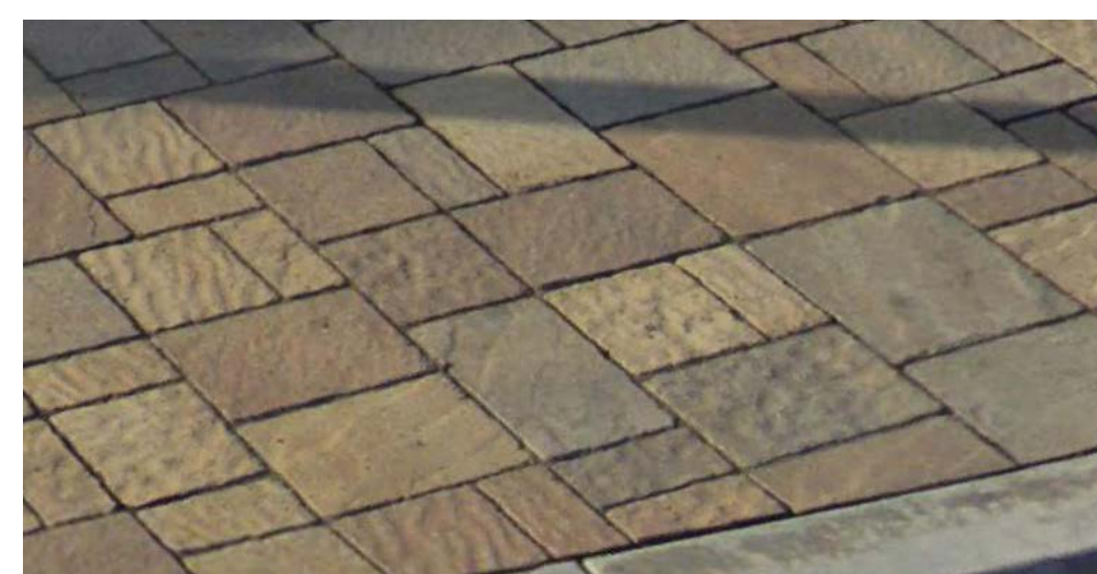
PERMEABLE CONCRETE PAVERS (TO MATCH PAVERS AT PIER AVE. & MANHATTAN AVE. CORNER PLAZA)
