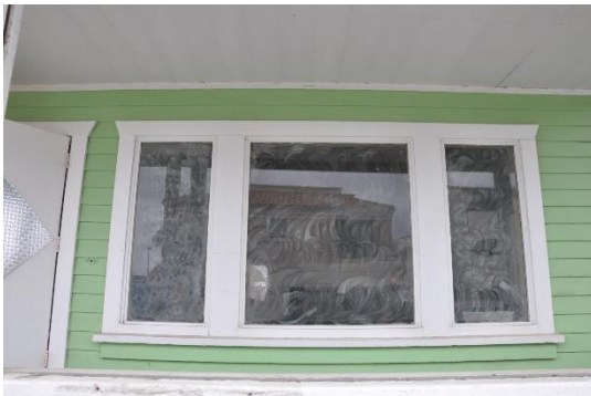
Figure 6: Tripartite window on each side of the main door with typical wood window surrounds that flare at the top.
