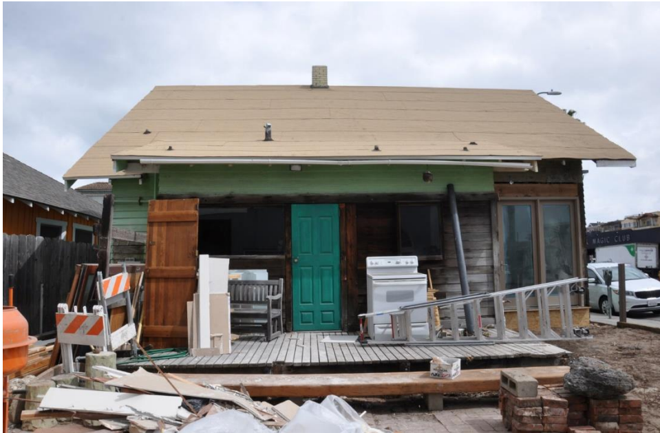
Figure 11: South (rear) façade with projecting section at the middle. View facing north.
